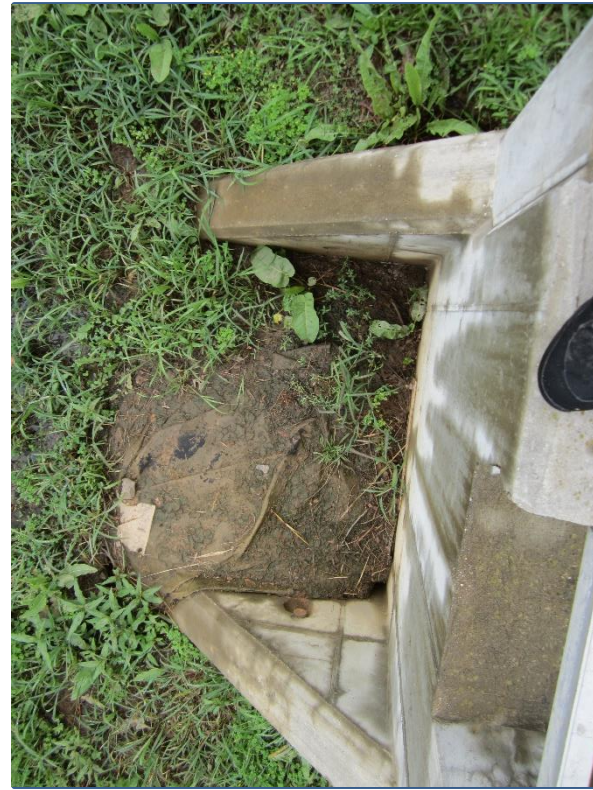
Outlet blockage by sediment
